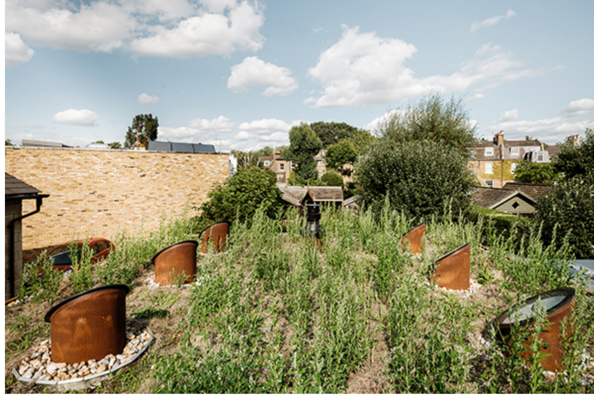
The planted green roof seen from the owners' bedroom with refurbished Corten roof glaze. Plants coming in!
